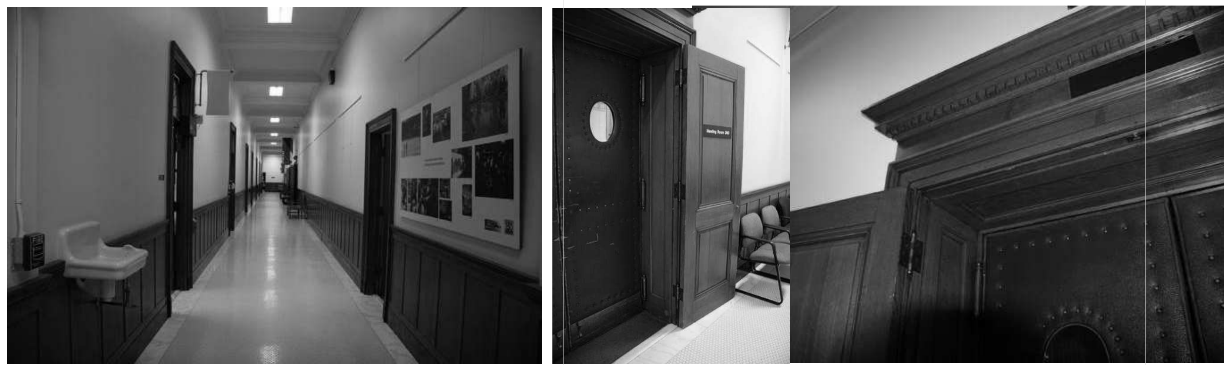
PHOTOGRAPHS OF THE EXISTING LEVEL 2 HISTORIC CORRIDOR AND ROOM 260 ENTRY DOORS FROM CORRIDOR SIDE
